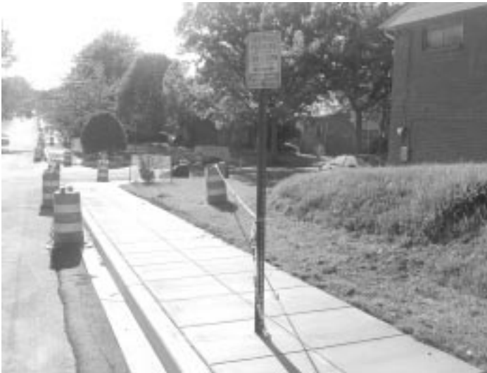
Does this make sense? Construction workers elected to leave the parking signs where they were before the sidewalks were installed, impeding pedestrian traffic.
