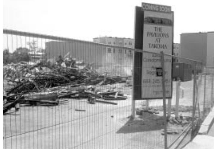
Construction of the Takoma Pavilions Complex in the 7000 block of Blair Road has begun. The picture, shown on the right, was taken on June 7, 2007.
